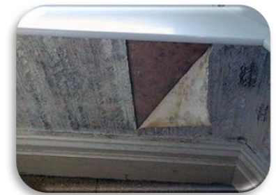
An example of serious condensation
